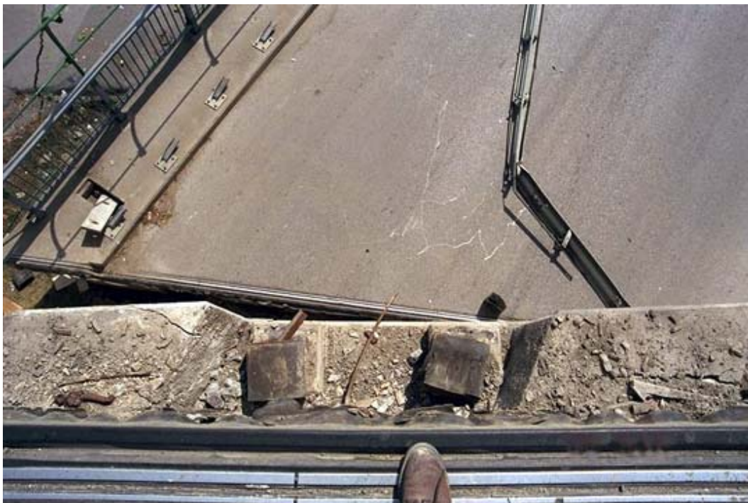
Figure 1-6 Unseating of the simply supported span from the abutment-mounted bearings
