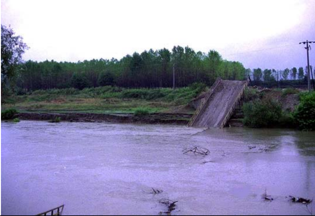
Figure 1-7 Collapsed and submerged bridge near Akyazi
