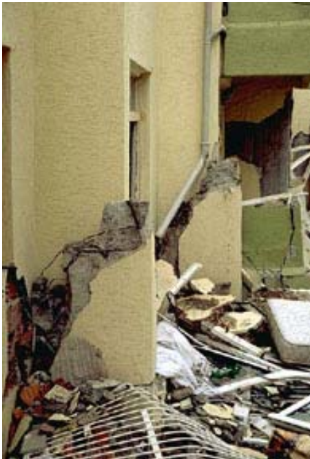
Figure 3-33 Damage to moment-frame columns
