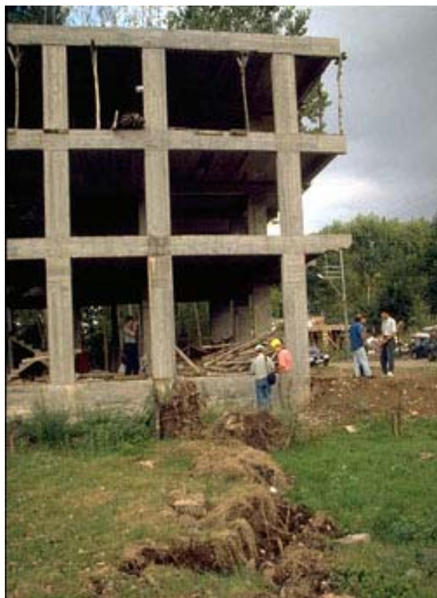
b. east-west elevation showing fault rupture
