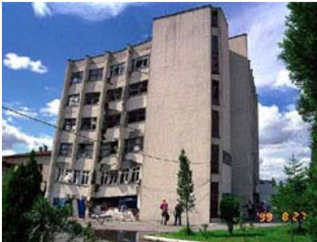
Figure 3-42 a. Damaged wall-frame building due to ground failure and wall rotation
