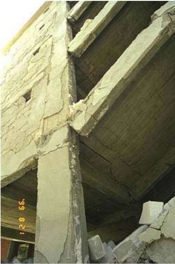
Figure 3-24 Damage to a nonductile reinforced concrete beam
