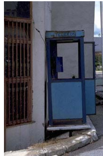
Figure 3-42 b. shear wall settlement
