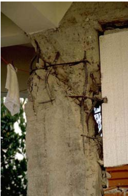
Figure 3-27 Shear failure of a moment-frame blade column
