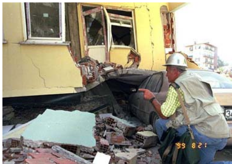
b. View of failed first story
