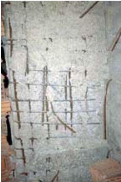
Figure 3-2 Poor quality construction of a shear wall in an apartment building in Yalova
