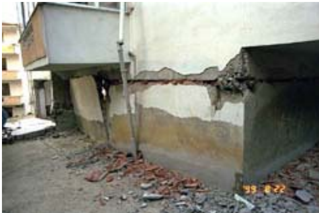
a. damage from out-of-plane deformation
