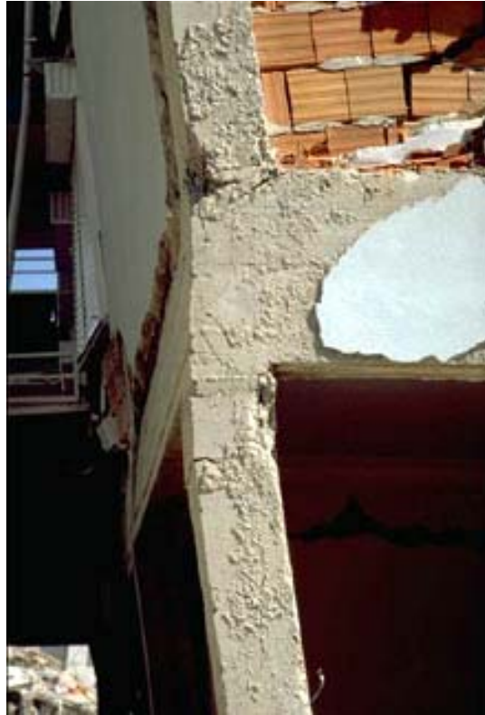
Figure 3-31 Concentrated damage at ends of moment-frame columns due to excessive drift
