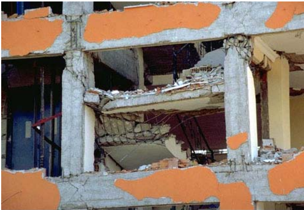
Figure 3-48 Damage at the rear stairwell
