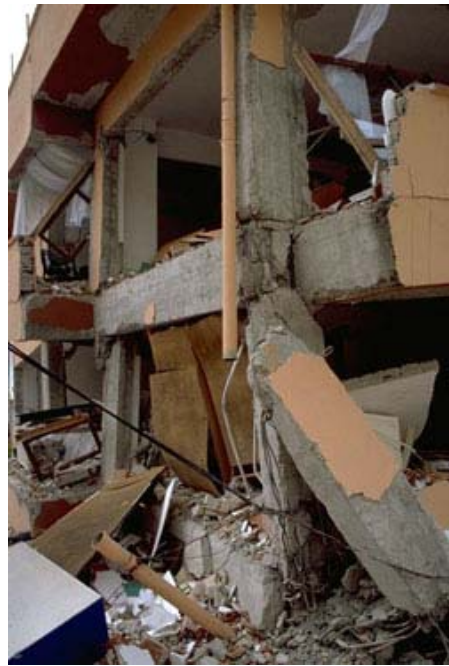
Figure 3-34 a. Damage to moment-frame beam-column joints
