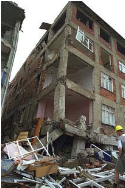
Figure 3-35 a. Building collapse due to failure of beam-column joints
