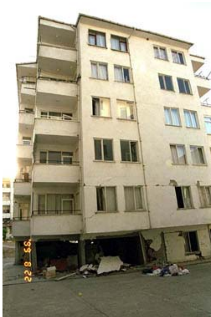
b. infill wall damage in Degirmendere
