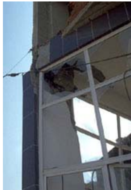
Figure 3-58 Damaged beam-column joint at top of first-story corner column, Building C.
