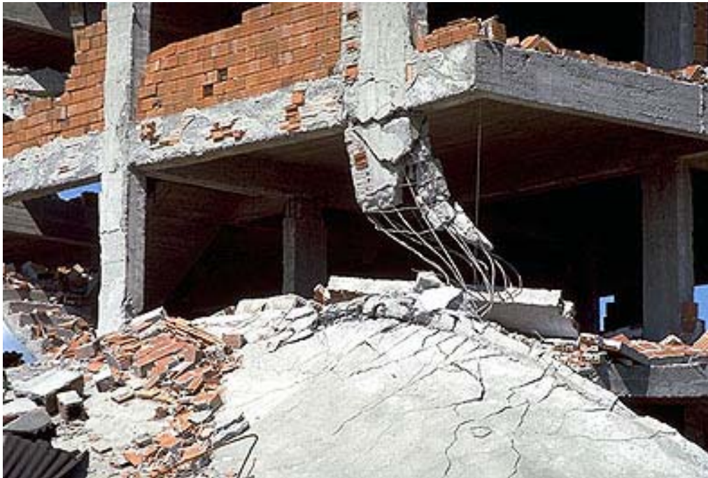
Figure 3-53 Details of damage to third-story column of Building B
