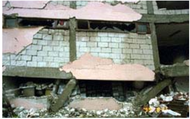
Figure 3-41 b. Close-up of failure of the shear wall and perimeter columns
