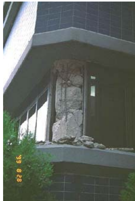
Figure 3-28 Lack of transverse reinforcement in moment-frame column
