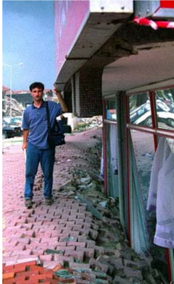
Figure 3-60 Settlement of Building D due to liquefaction and soil-bearing failure
