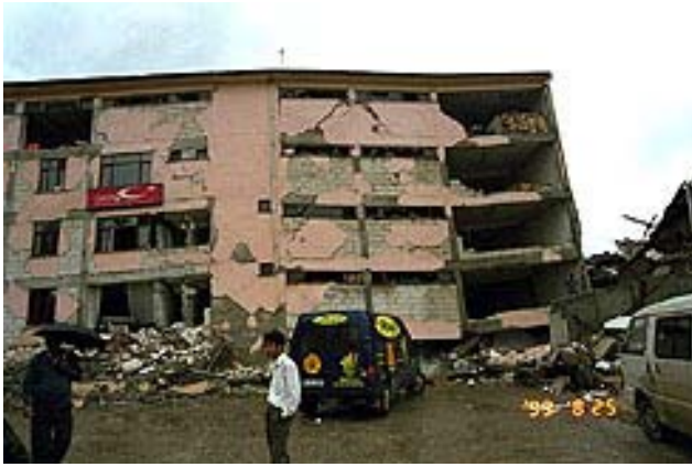
Figure 3-41 a. Collapse of dual wall-frame five story building, Adapazari
