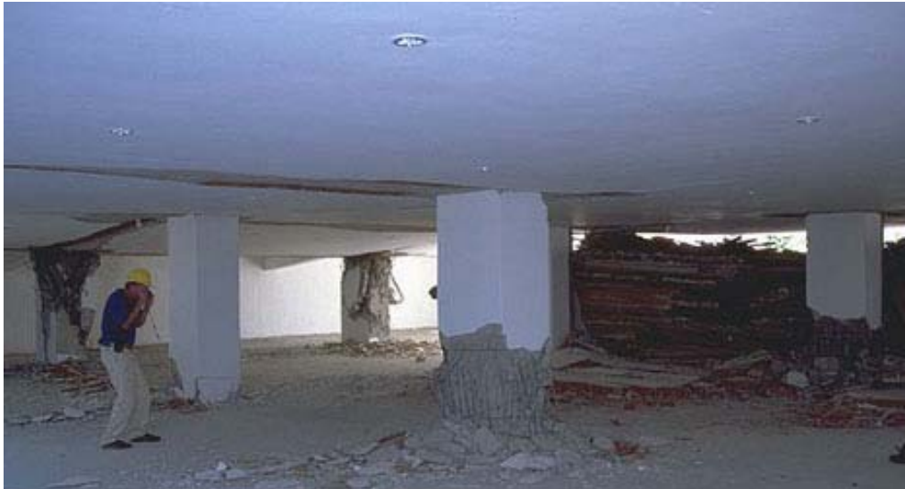
Figure 3-47 Damage to first story columns
