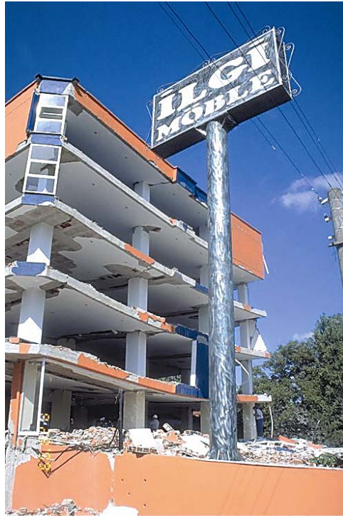
Figure 3-37 Typical damage to asmolen floor systems
