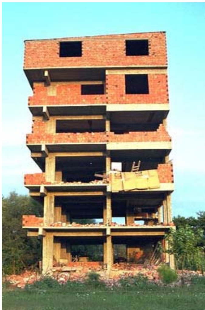
a. infill wall damage in Gölcük
