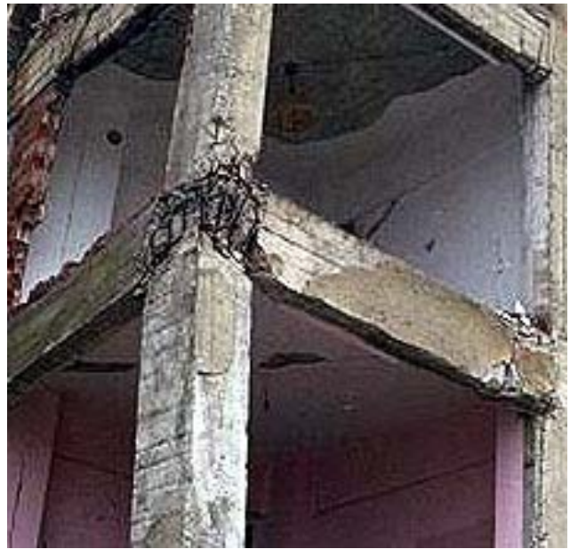
Figure 3-35 b. Damage to one beam column joint
