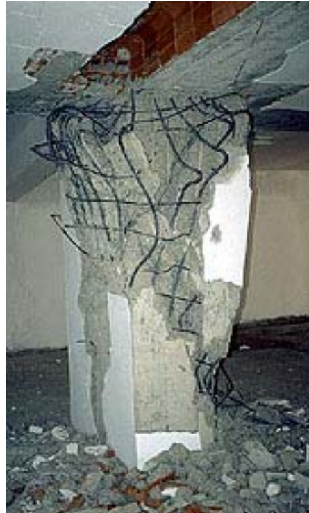
Figure 3-50 Axial failure of column B (See Figure 3-46)
