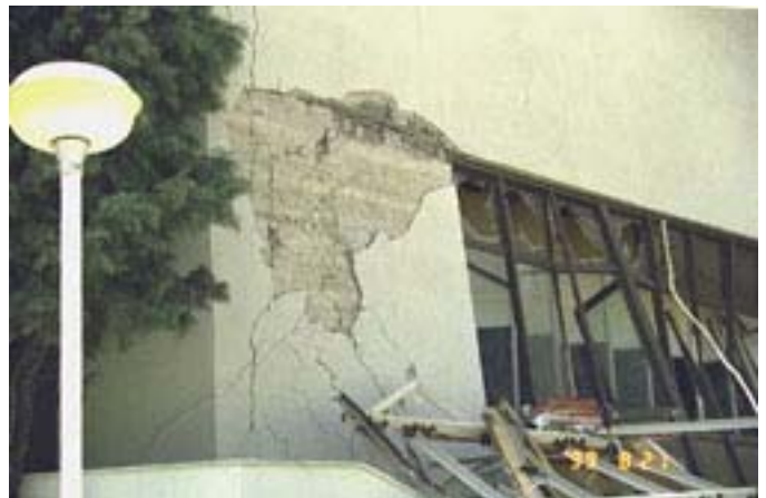
Figure 3-40 b. Close up of damage to a shear wall
