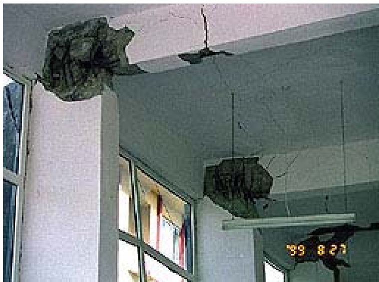
Figure 3-36 Damage to a new moment-frame beam-column joint
