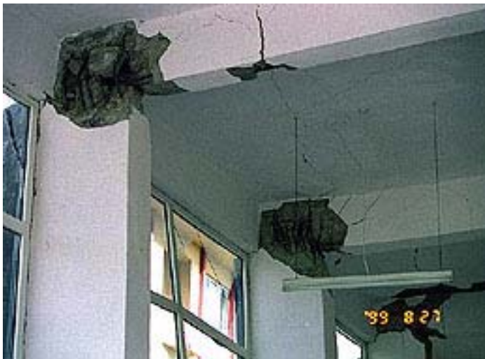
Figure 3-57 Damaged beam-column joints at top of first story columns, Building C
