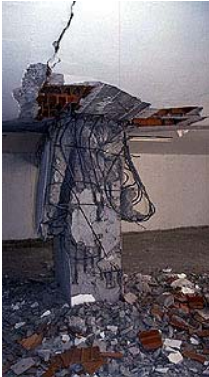
Figure 3-49 Shear failure of Column A (See Figure 3-46)
