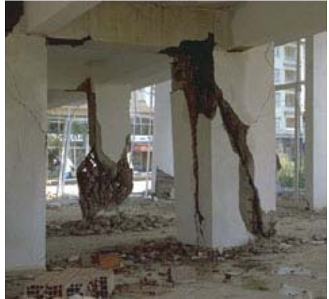
Figure 3-56 Shear crack in the first story column in the rear of Building C
