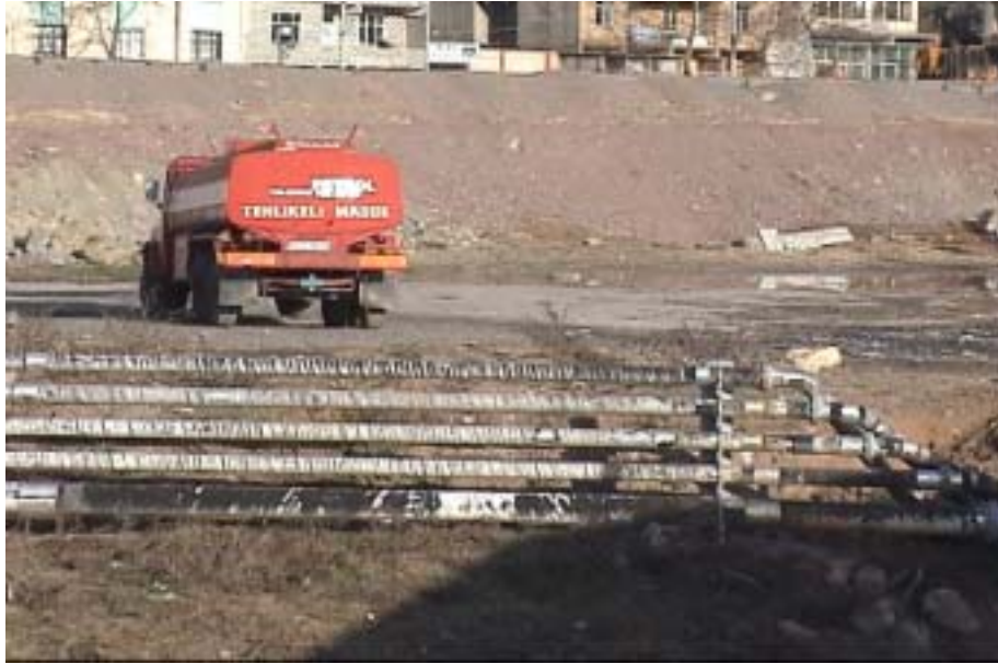
Figure 3.2.39. Crude oil transmission lines in central Dilovasi
