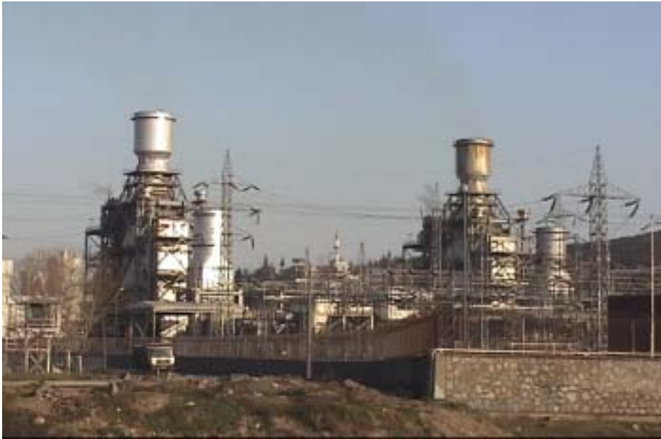
Figure 3.2.34. The 360 GWh/year capacity power generation-unit of Ova Electric Company fuel source: N.G.
