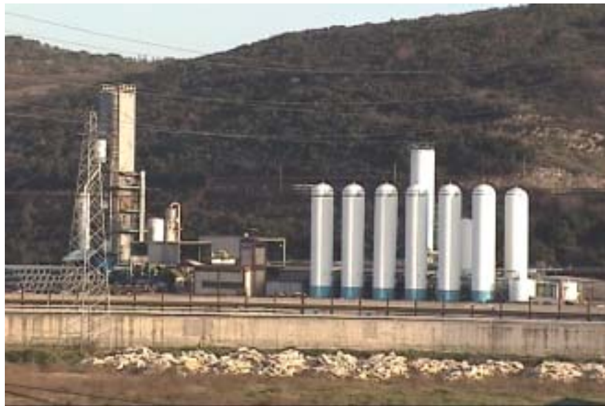
Figure 3.2.38. Vertical storage tanks in southern Dilovası. Foundation anchorages are susceptible to damage due to rocking motion during an earthquake.
