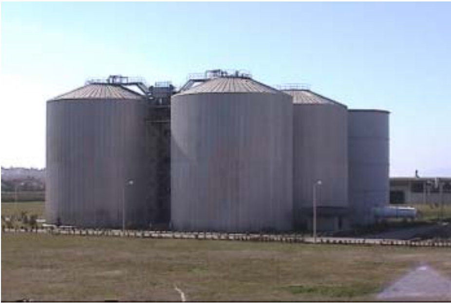
Figure 3.2.78. Closer view of the waste water treatment tanks.
