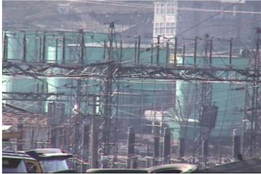
Figure 3.2.35. Electrical transmission and control equipments of Ova Electric company.
