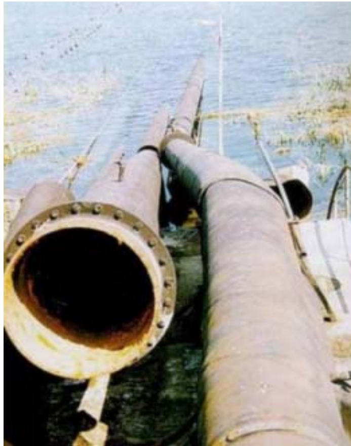
Figure 4.18. Damaged water pipes.
