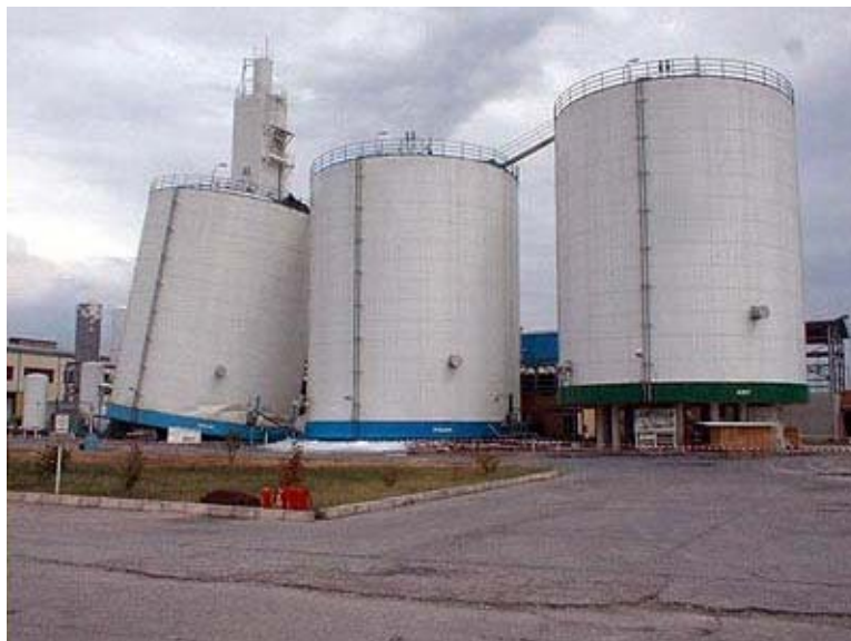
Figure 4.12. Damaged insulated tanks at HABAŞ Facility.
