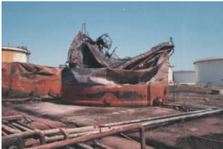
Figure 4.11. Fire caused buckling of a tank at TÜPRAŞ Refinery.
