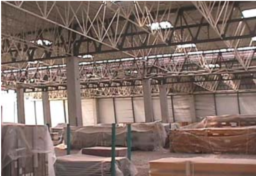
Figure 4.3. Damaged prefabricated building at Ford Otosan Plant.
