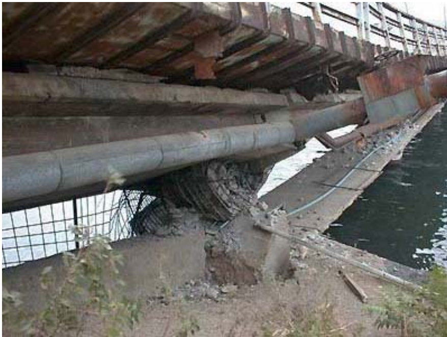
Figure 4.27. Failed supporting column at SEKA port.
