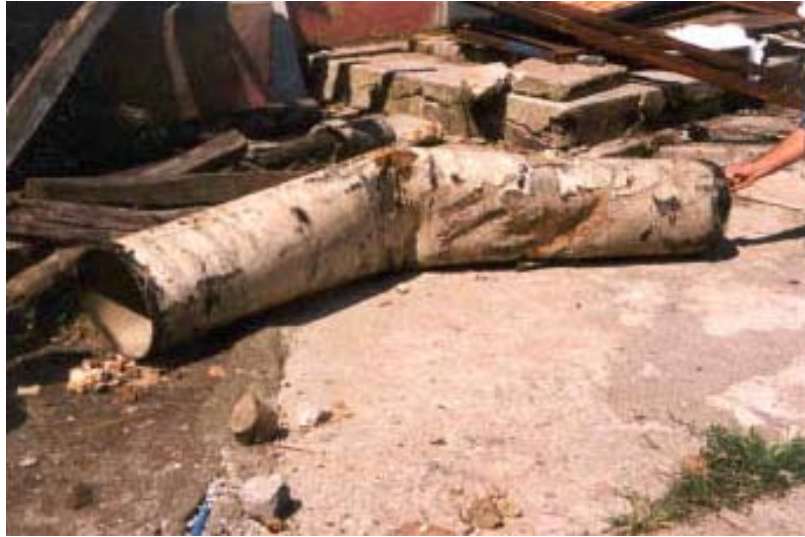
Figure 4.17. Steel pipe damaged due to fault effect at Arifiye.
