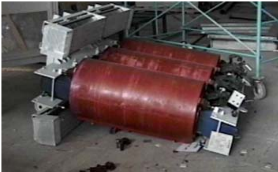
Figure 4.7. Damaged electrical equipment.
