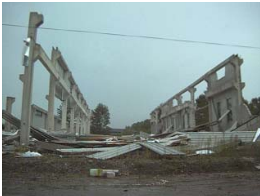
Figure 4.1. Collapsed prefabricated structure.
