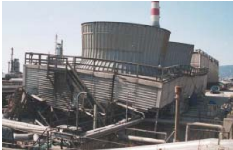
Figure 4.14. Collapsed cooling tower at TÜPRAŞ Facility.
