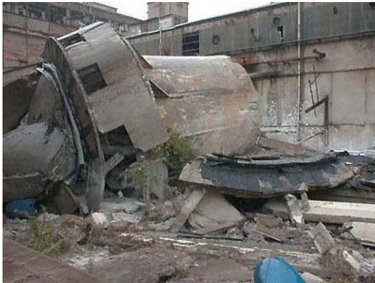
Figure 4.13. Collapsed silo at SEKA Paper Factory.
