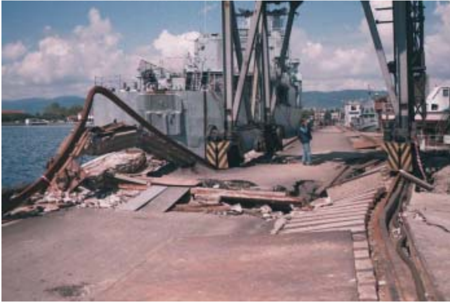
Figure 4.22. Damage at navy port in Gölcük.
