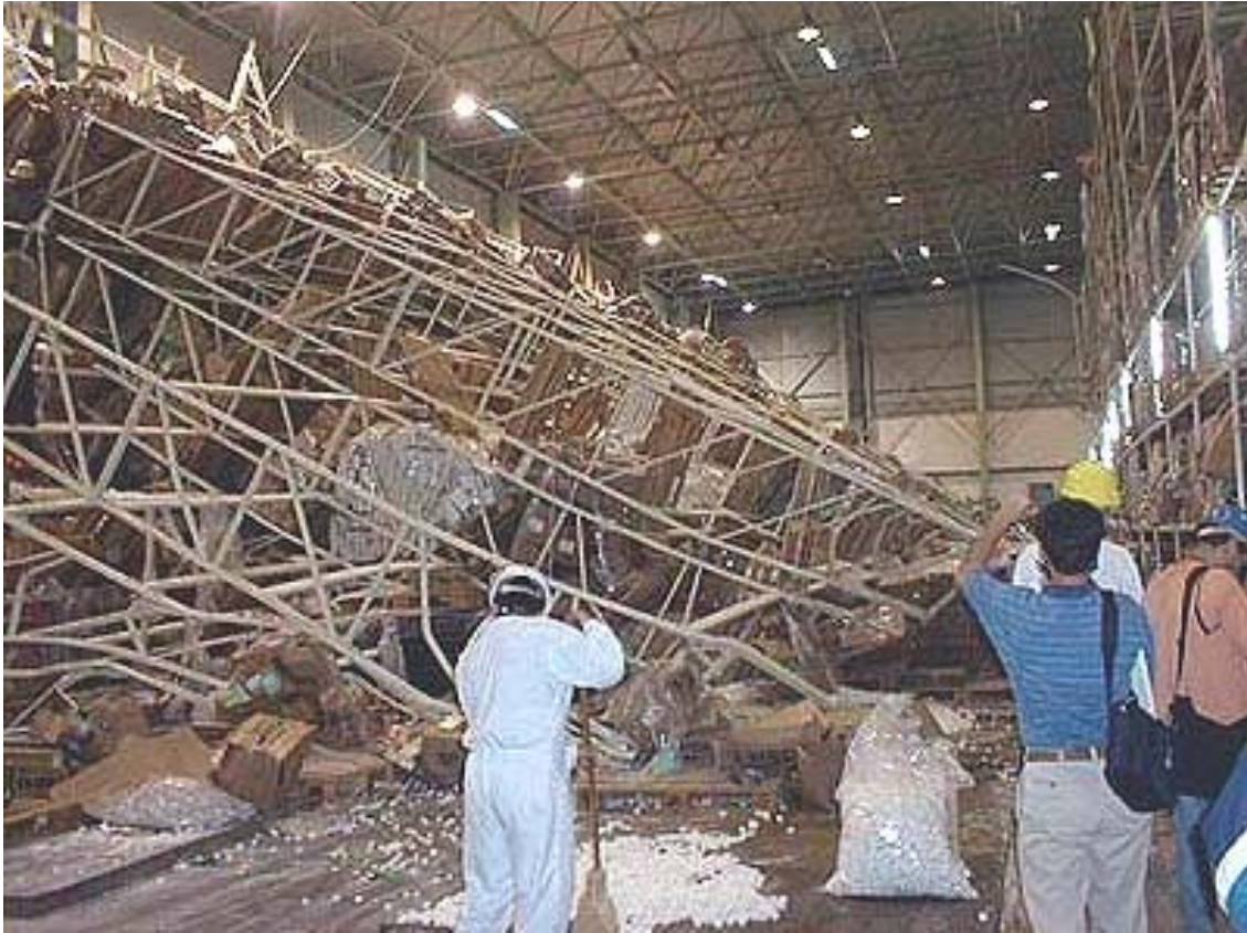
Figure 4.32. An example of industrial facilities experienced losses of rock-stored items in buildings.
