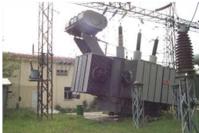
Figure 4.6. Damaged transformer at Izmit-1 substation.
