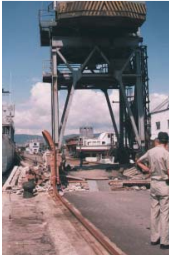
Figure 4.21. Crane and rail damage at Gölcük navy port.
