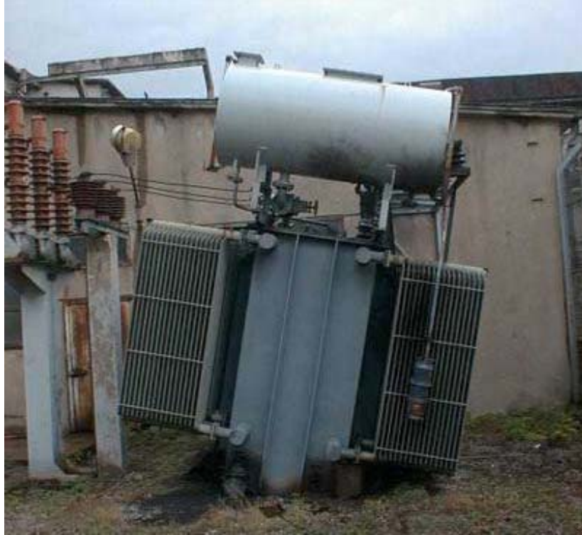
Figure 4.8. Damaged transformer at SEKA paper factory.
