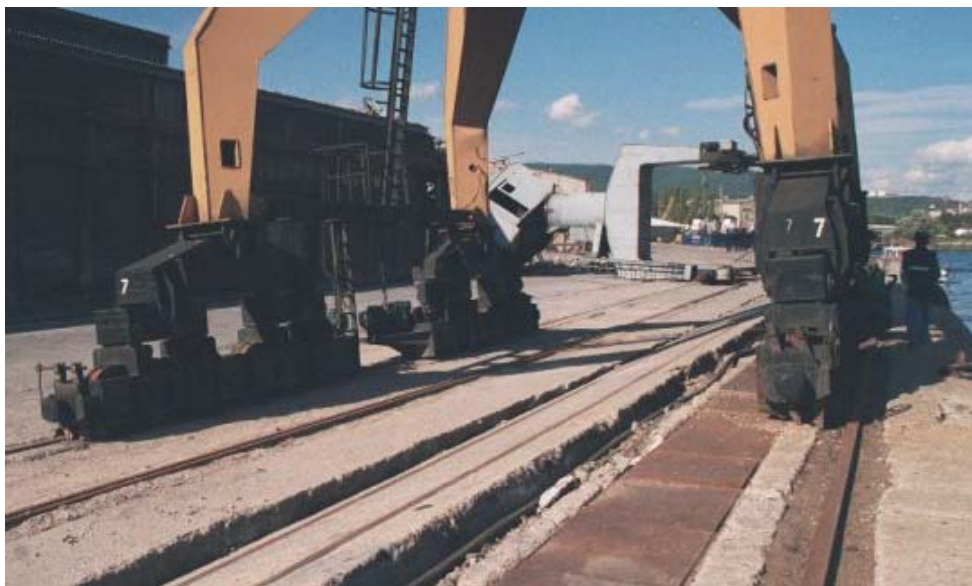
Figure 4.24. Damage at Derince Port in Kocaeli Earthquake.
