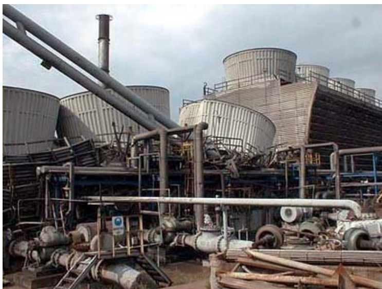
Figure 4.15. Collapsed cooling tower at PETKİM Facility.
