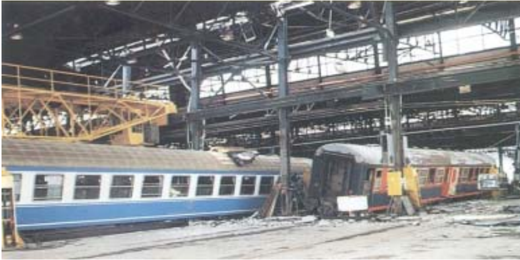
Figure 4.4. Damaged steel structure at Adapazari rail car factory.
