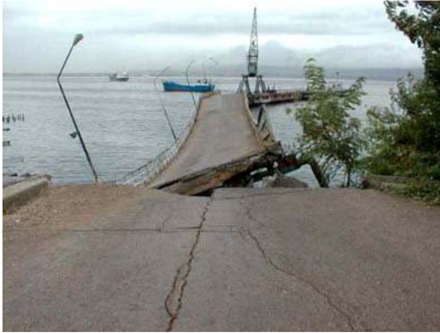
Figure 4.28. Damage at SEKA pier.
