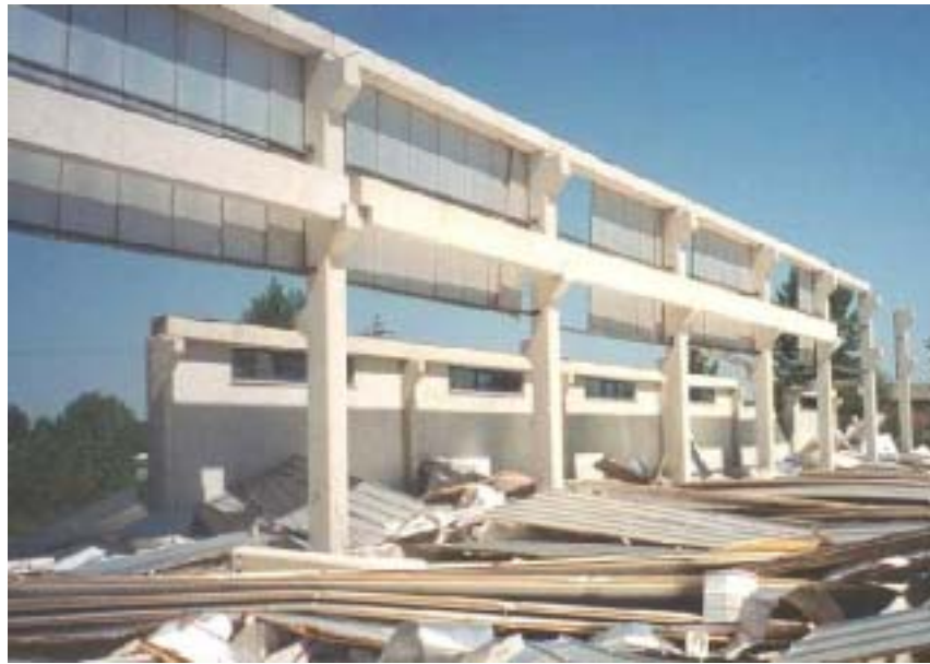
Figure 4.2. Damaged prefabricated frame system.
