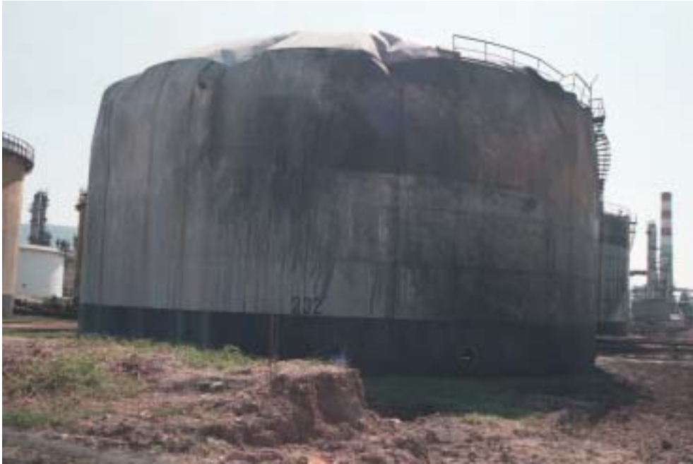
Figure 4.10. Tank failure at TUPRAS Refinery due to fire caused pressure increase.
