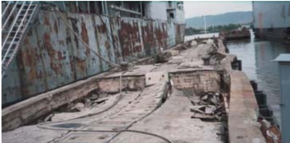
Figure 4.23. Damage at navy port in Gölcük.
