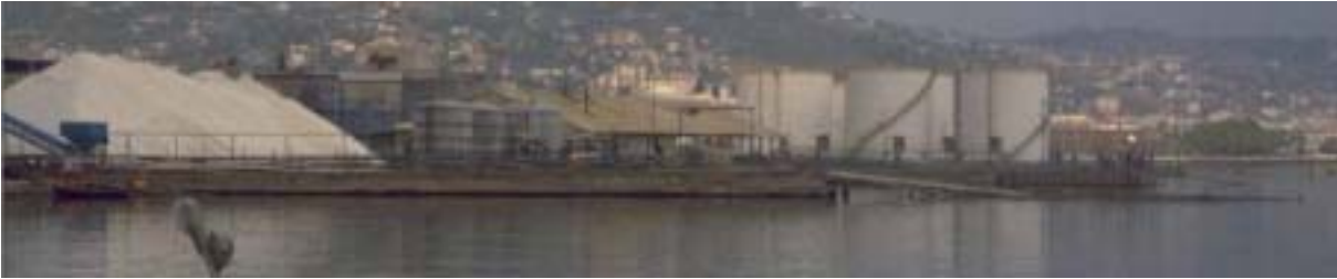
Figure 4.26. Damaged pier at Shell and Trans Turk facilities.
