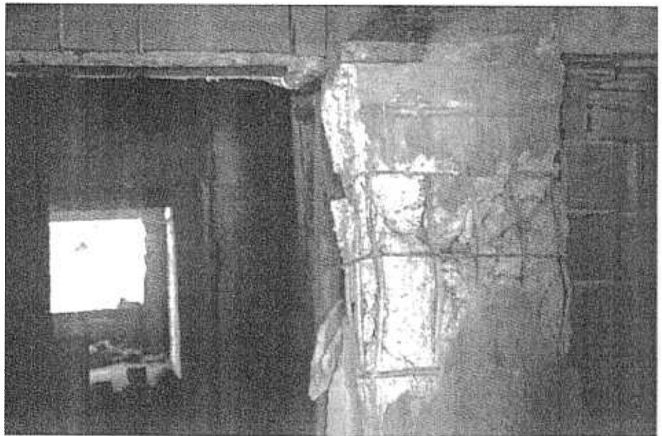
Figure 9 - Typical strong-axis column shear failure.
