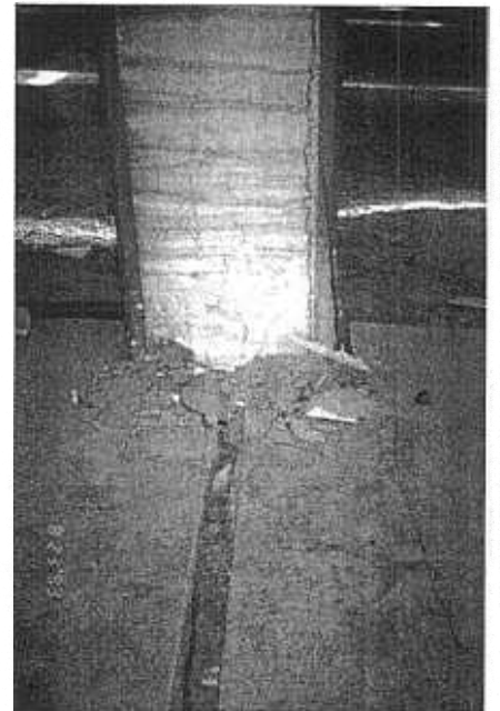
Figure 3 - Column pushed through the floor slab and tilted due to 0.5 right-lateral fault displacement. Column underwent ductile deformation without losing significant axial load capacity. (Photo: Youd)
