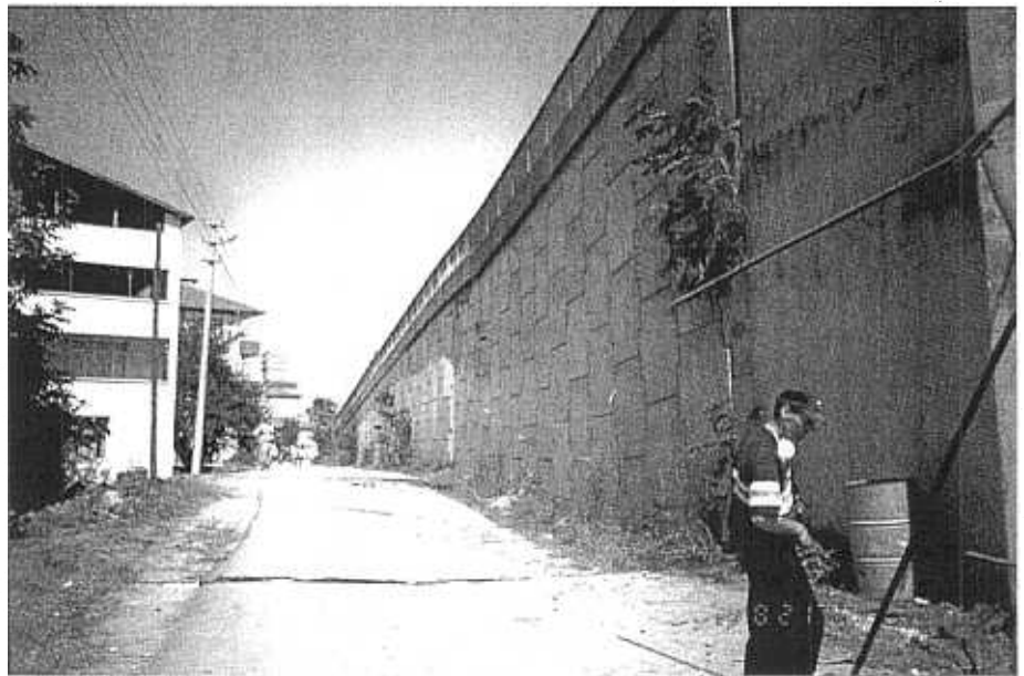
Figure 5 - Mechanically stabilized earth wall within a few meters of the primary fault rupture. Although subjected to differential settlement, it suffered only minor damage. (Photo: Youd)
