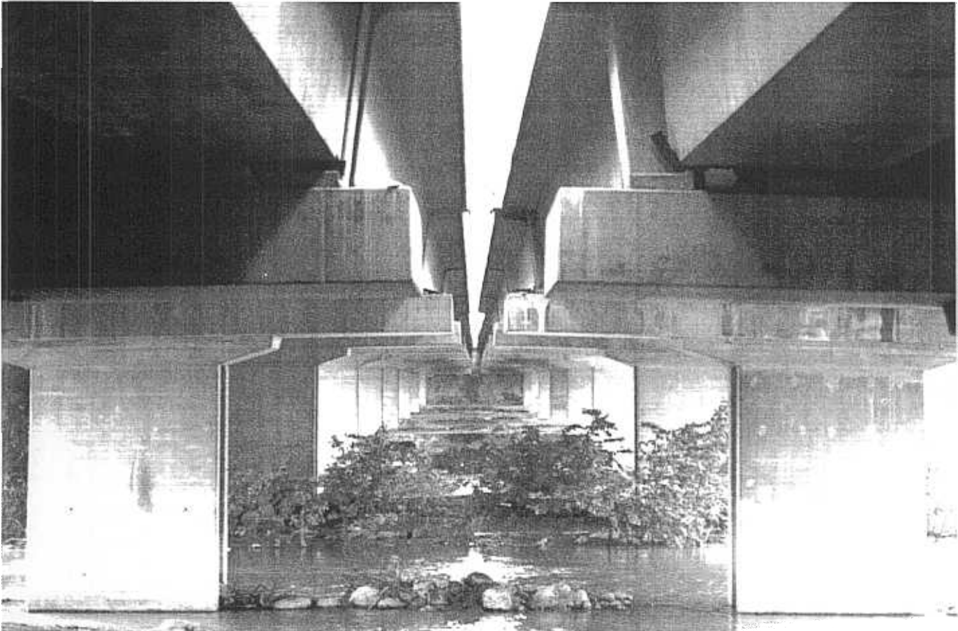
Figure 11 - The east (left) and westbound bridges over the Sakarya River. Note shifting of the spans and the unseating of the bearings in the westbound bridge. The bearings on the eastbound bridge have partially "walked out," but not unseated. (Photo: Mander)
