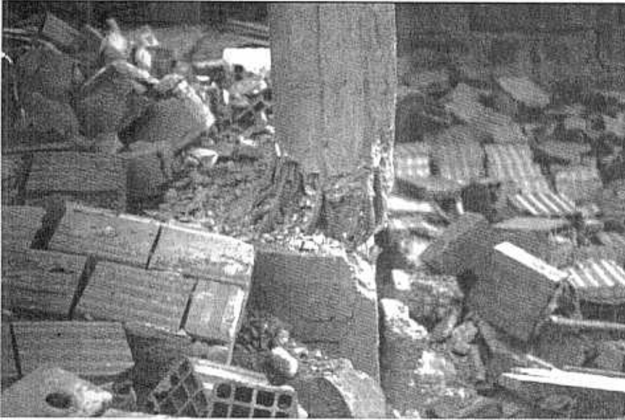
Figure 8 - Typical weak-axis column hinging.
