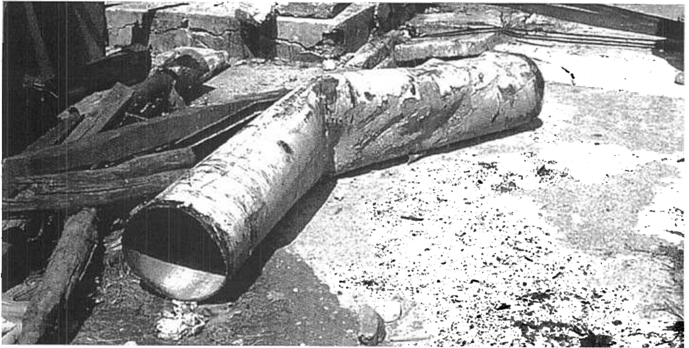
Figure 12 - Buckled steel pipe at crossing near Arifiye.
