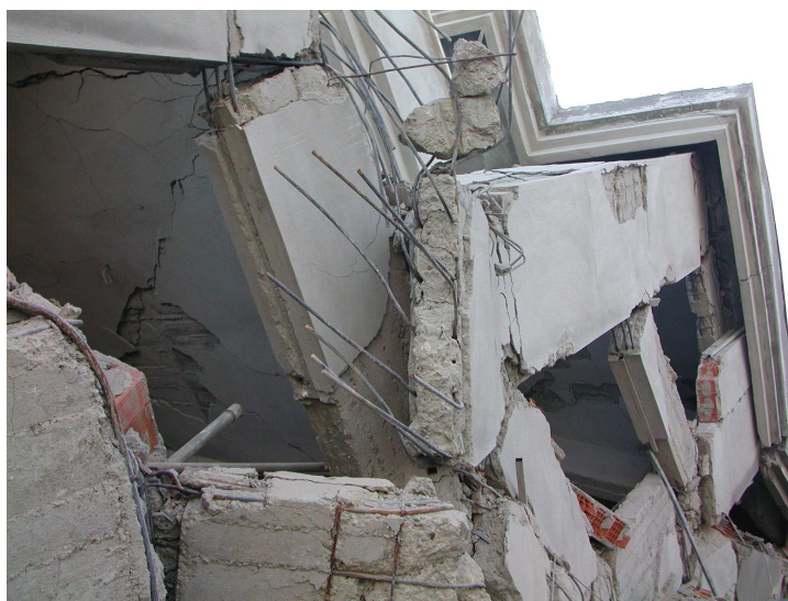
Photo 9.1.3 An example of the failure between the column and the beam
