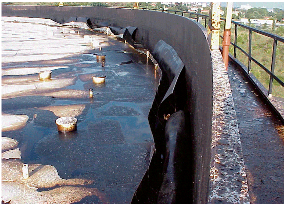
Figure 4: Damaged seals in tanks from sloshing of liquids
