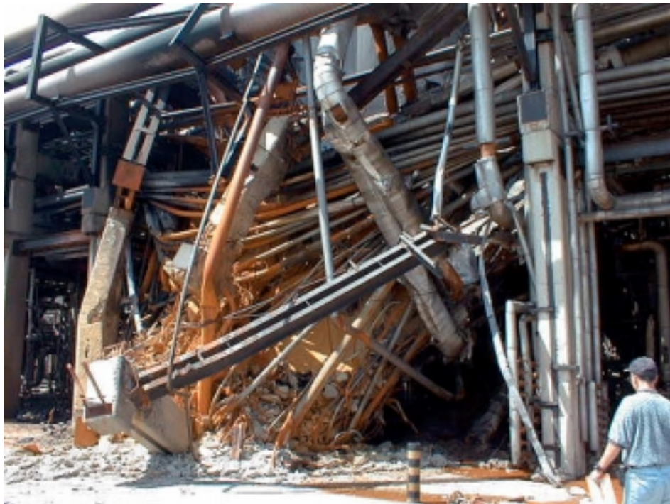
Figure 7: Lower part of collapsed stack fell into pipeway, destroying pipes and structure, causing fires
