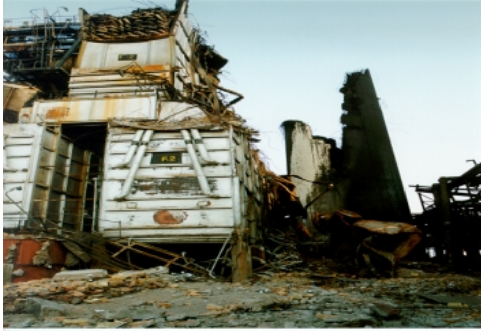
Figure 6: Collapse of stack inside crude unit damaged large heater
