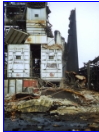
Figure 6: Stack collapsed in Crude Unit
