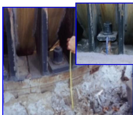
Figure 8: Damage at the base of reactor vessel
