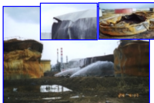
Figure 5: State of damage to tanks
