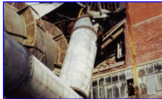
Figure 12: Steel stack collapsed into processing unit
