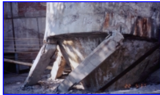
Figure 9: Collapsed silo at Seka Paper Plant
