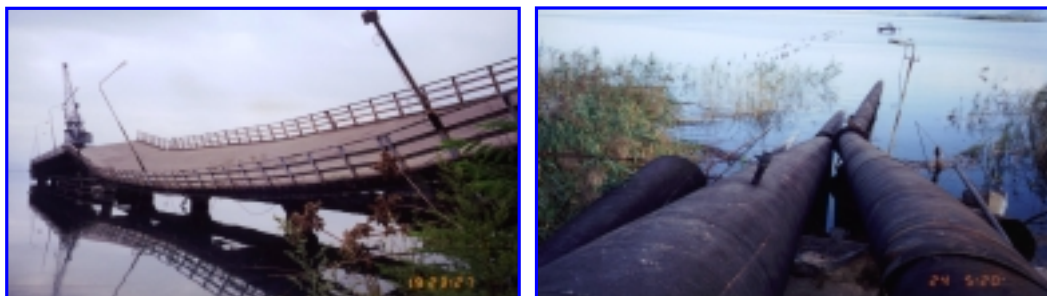
Figure 10: The collapse of wharf deck at Seka paper plant and collapse of pipeline at pump station
