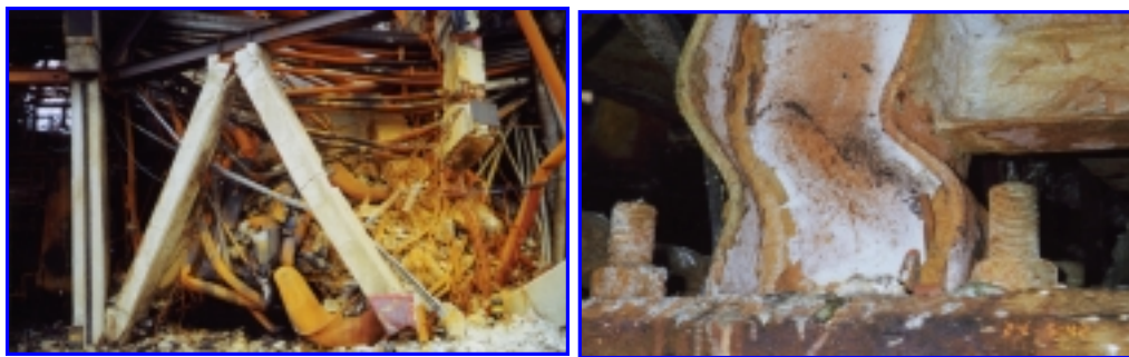
Figure 7: Destruction of the piping system and buckling of steel columns supporting furnace
