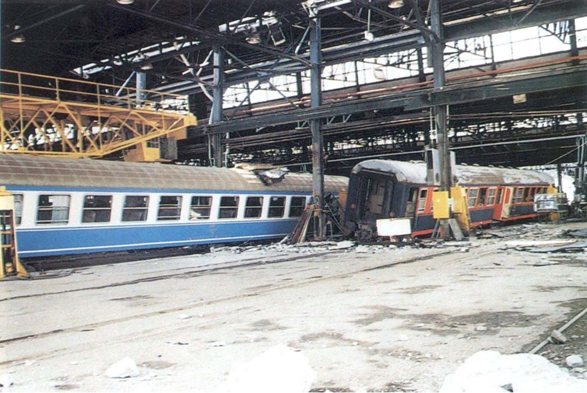
Adapazari rail car factory, damaged steel frame
