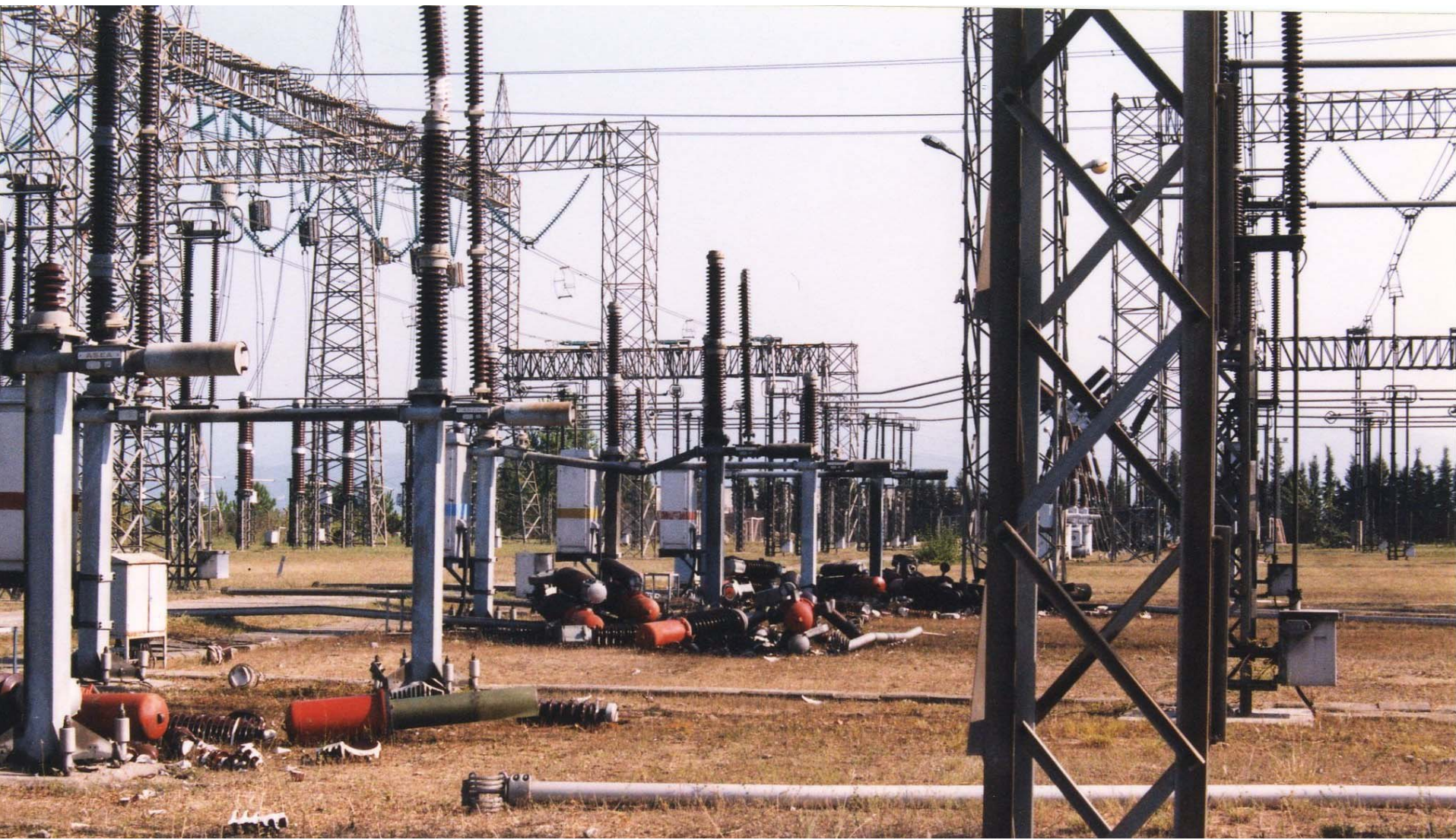
Adapazari 380 kV Substation
