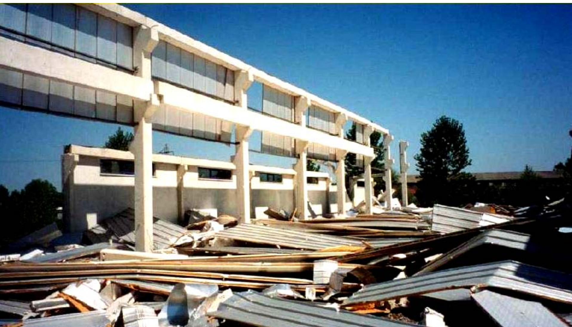
Damage to prefabricated factory buildings
