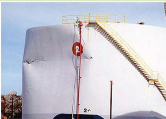
Figure 4. Tank damage caused by hurricane winds (Source: AIR)
