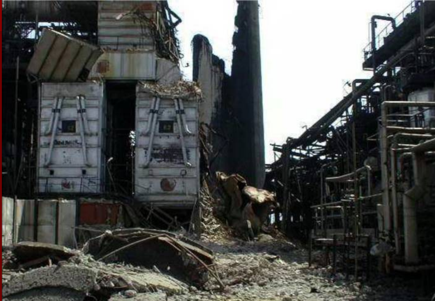
TÜPRAŞ, Fallen Stack
