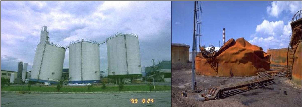
Figure 21a-b. (a) Sloshing damage to upper shell of tank (left), Elephant-foot buckling of the tank wall. (b) yielding of the support structures (left), collapse of the tank (right).
