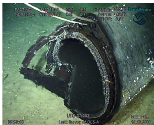
Figure 11.4 Picture of the ruptured loading hose
